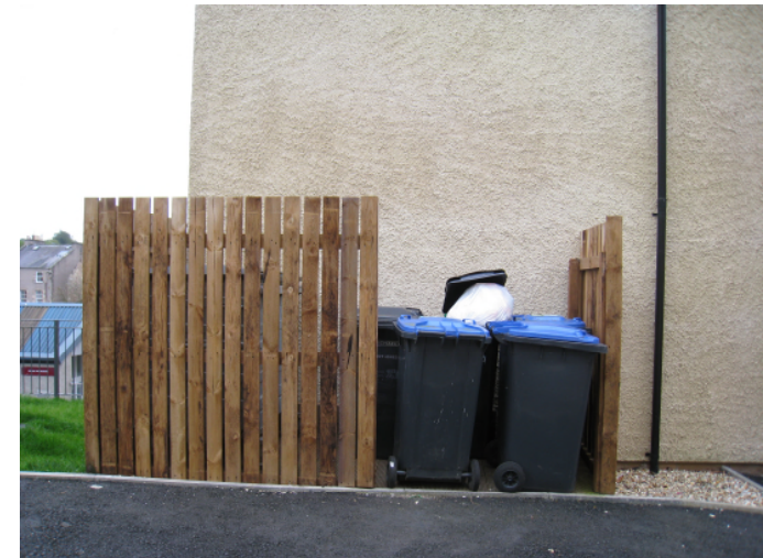
Example of bin storage area which is too small, not allowing sufficient space for filling and emptying bins
