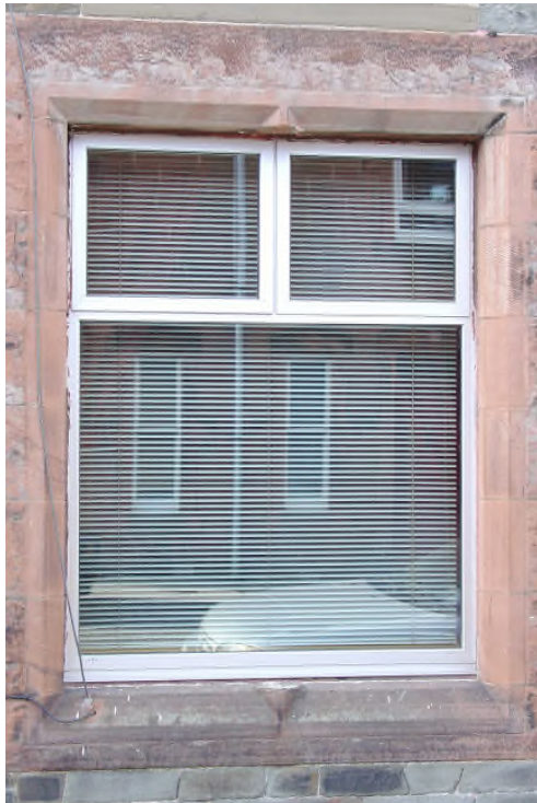
Figure 19: Replacement Window, which removes the central mullion and changes the whole character
