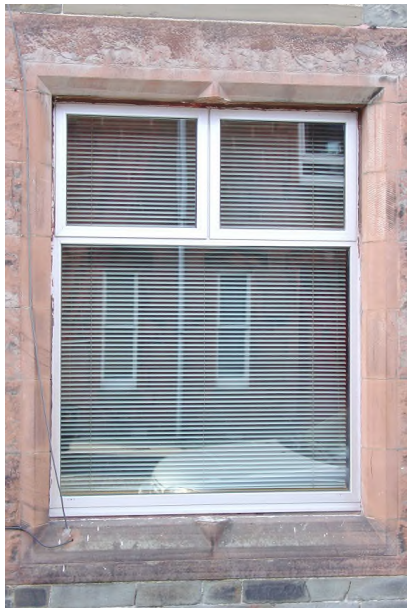
Figure 18: Replacement Window, which removes the central mullion and changes the whole character of the window opening.
