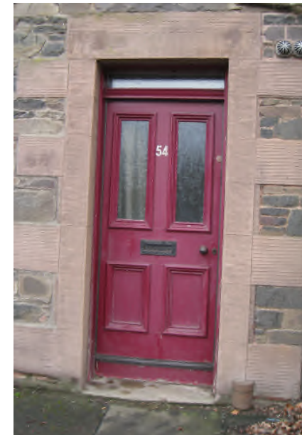
Figure 26: Door Alteration - Replacement of upper timber panels with glazing to allow additional light internally.
