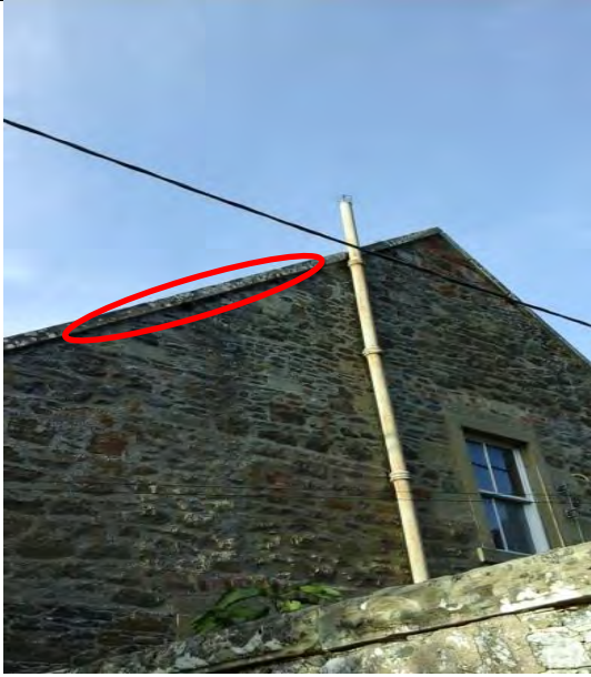
Building with High BRP. Gaps under roof
