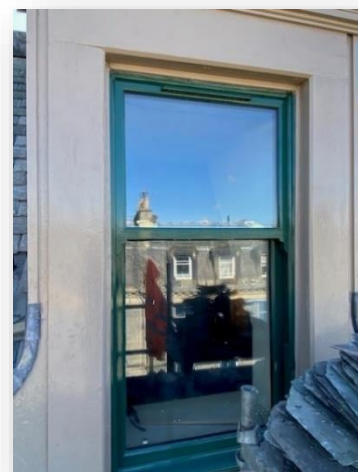
Completed lead work to the turret and window repairs at 80 High Street
