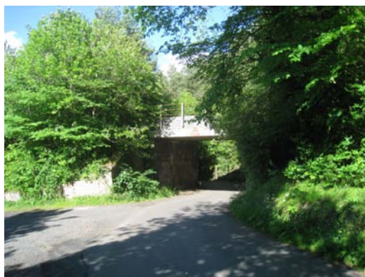
The old railway bridge over Whitelee Road – an umbilical cord linking the Southern Expansion area with the village centre.
