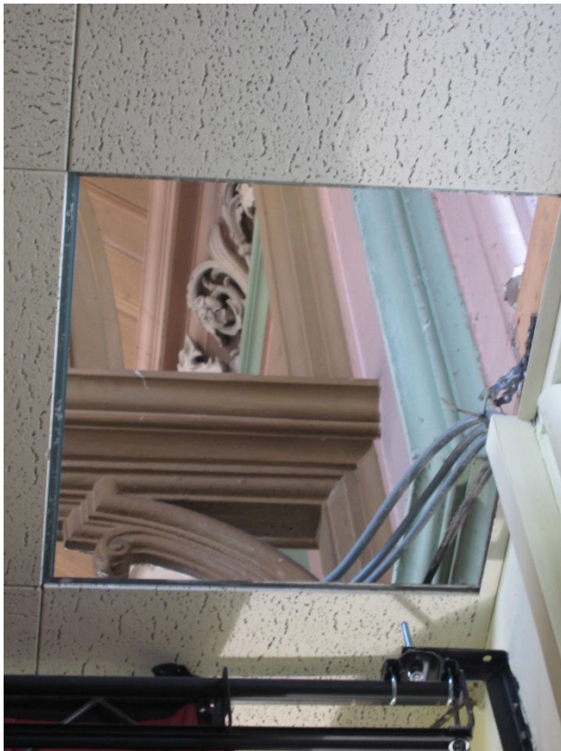
View through the suspended ceiling of the Burgh Hall showing the ceiling / roof structure beyond
