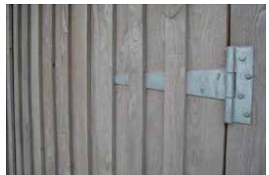
Figure 5 : 70 x 18mm on 150 x 18mm with 80mm gap on front face, off saw, stained. Used here to make timber shed doors.
