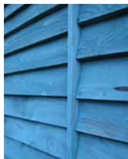
Figure 9 : 150 x 20mm straight edged boards simply overlapped horizontally, with a face of 135mm, off saw, painted.
