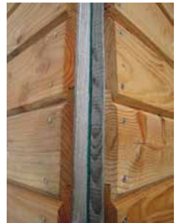
Figure 12 : 125mm finished face, 20mm deep, fully profiled and dressed boards, before corner piece installed.
