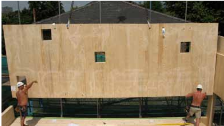
Cross glue laminated solid timber panels are a type of massive timber that is widely used throughout Europe and Scandinavia. Here, an entire wall of one storey is being craned into place for a house in London. Architect: David Adjaye. Photo: Eurban
