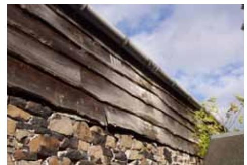
Figure 10 : 25mm depth off saw elm boards with one waney edge, simply overlapped horizontally and treated with creosote.
