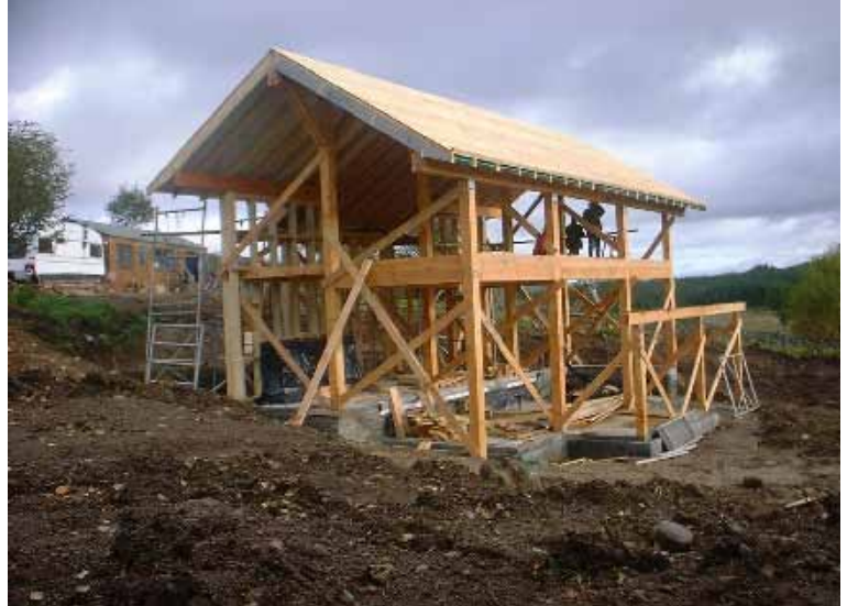
A post and beam frame designed by Neil Sutherland Architects in Scottish Douglas fir under construction. Photo: Neil Sutherland Architects
