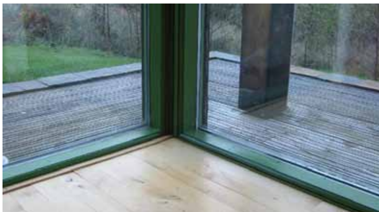
Floor of home grown ash, sourced and machined in the Highlands by Neil Sutherland Architects. Photo: Bernard Planterose
