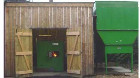
Industrial scale wood chip boiler producing heat only Buccleuch Estates, Selkirk
