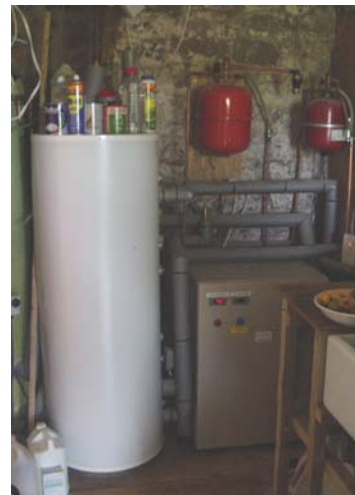
Heat exchanger and distribution system
